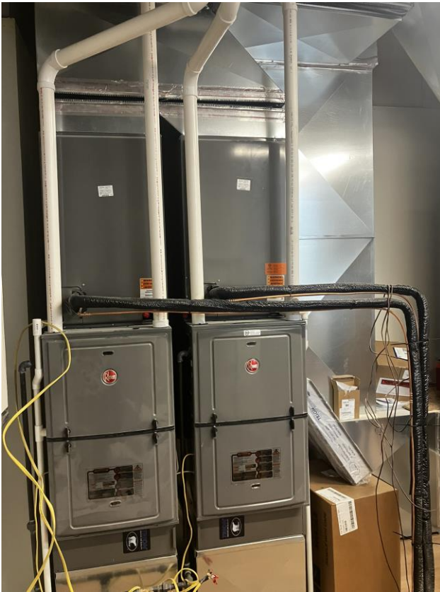
12. Mechanical Units in Furnace & Utility Room 114
