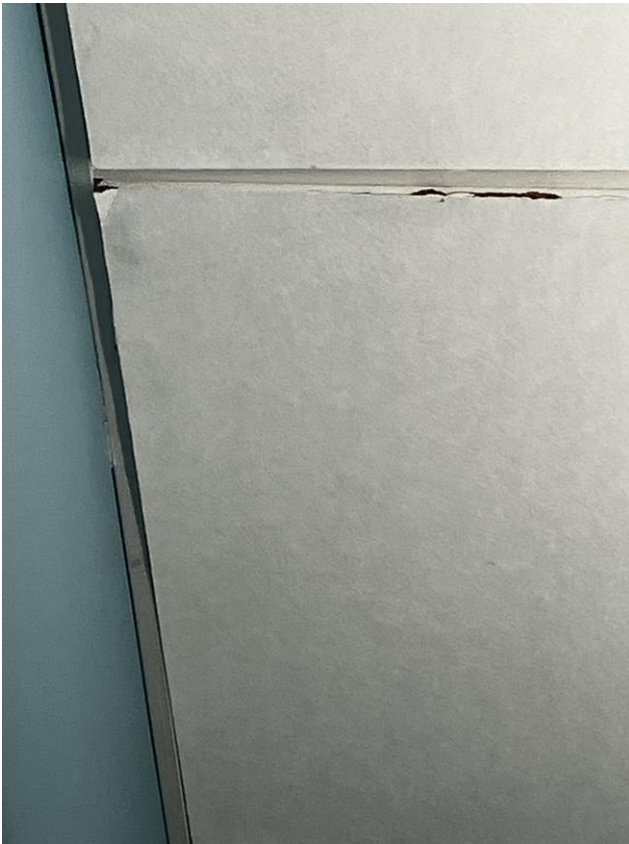
24. Example of Ceiling Tile Damage
