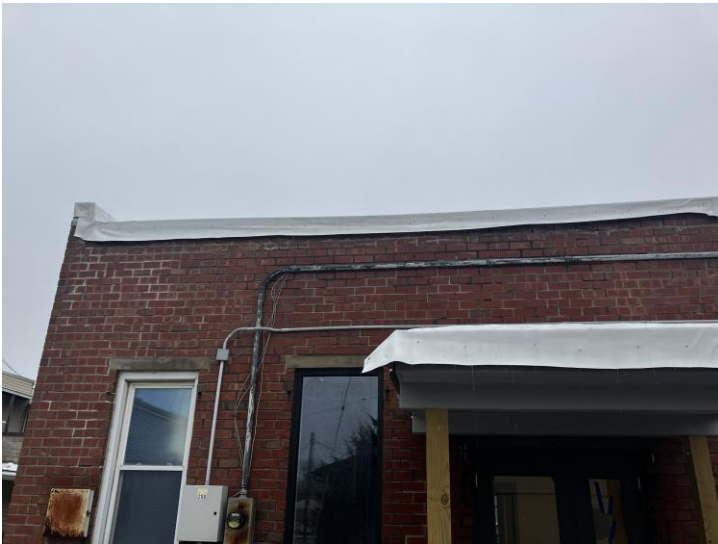
19. Rear Roof Edge, Missing Louver
