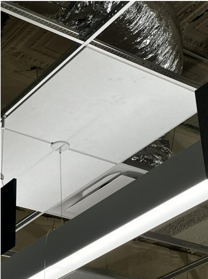
25. Example of Dirty Ceiling Tile
