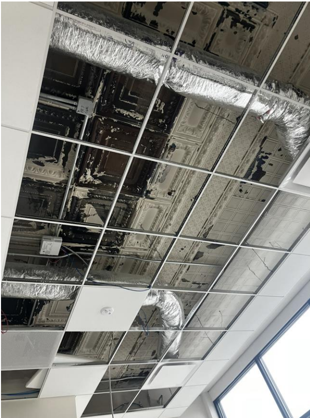
4. Example of Missing Ceiling Tiles
